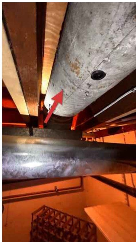
Ducting has asbestos tape
