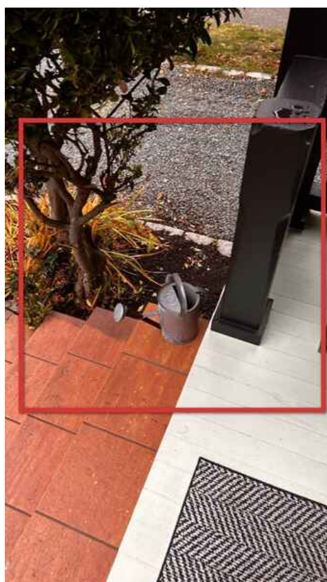
Potential Fall Hazard
