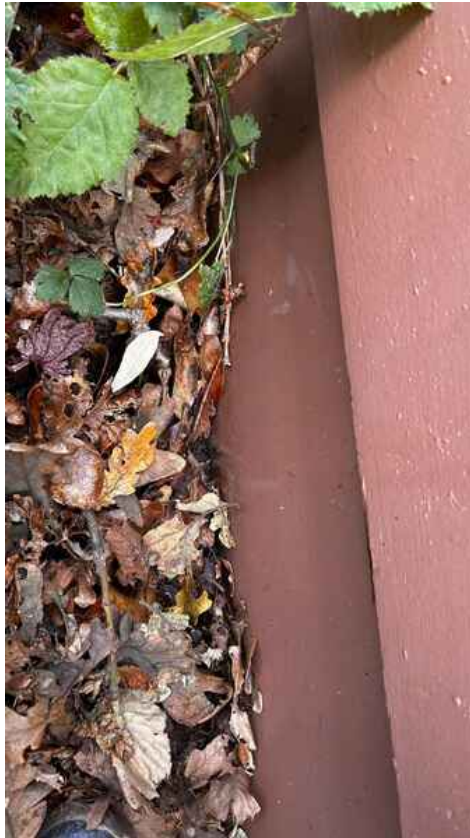
Siding too close to grade
