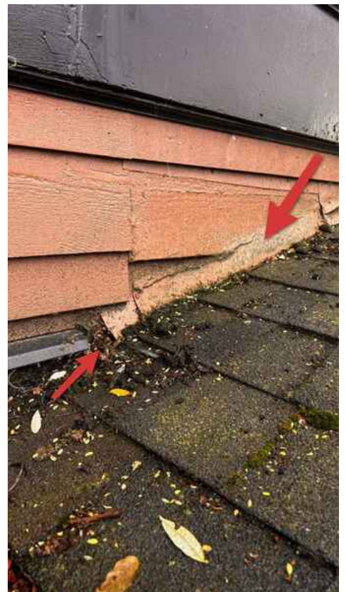
Flashing needs attention
