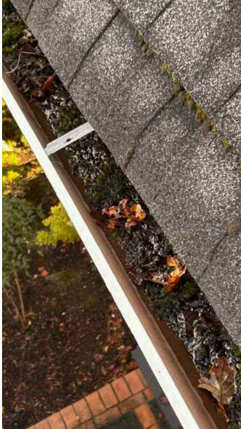
Moss and Debris in Gutter
