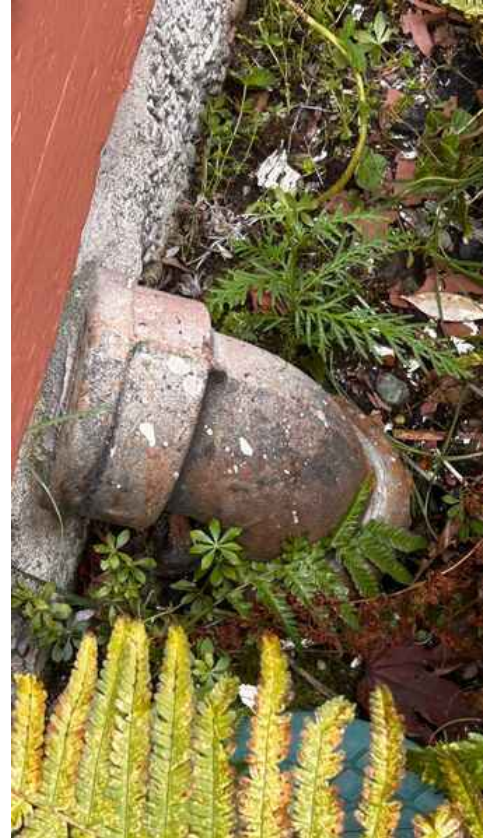
Cast Iron Drain Waste pipe
