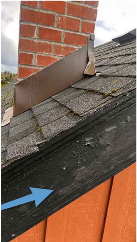
Peeling Fascia Paint
