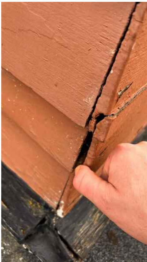
Loose corner joints
