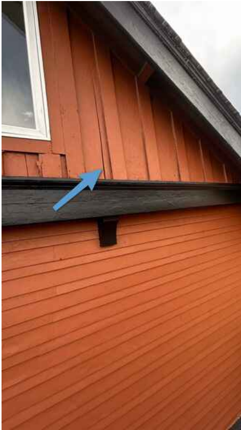
Cracked Siding board
