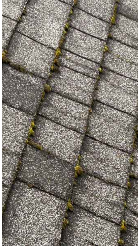
Granular loss and moss
