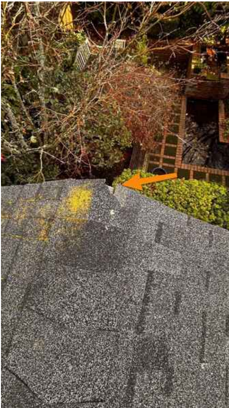
Torn Ridge shingle
