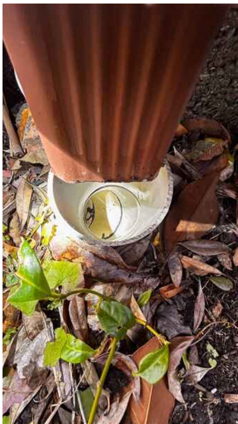
Grade nearly encroaching on riser
