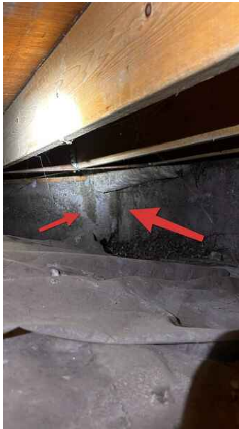
Moisture from corner
