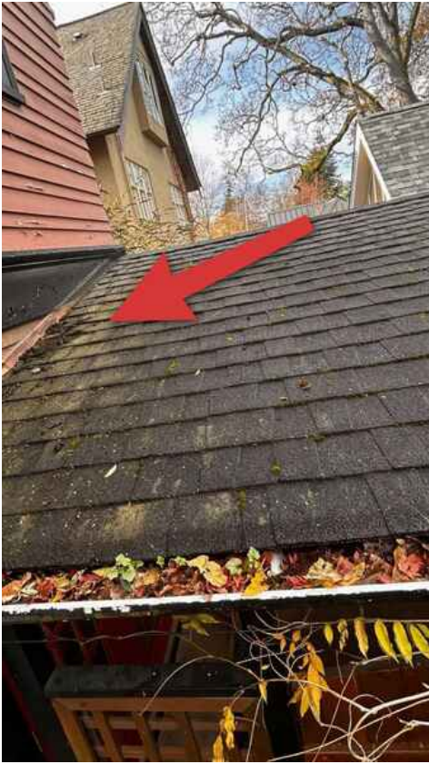
Possible racoon droppings on roof
