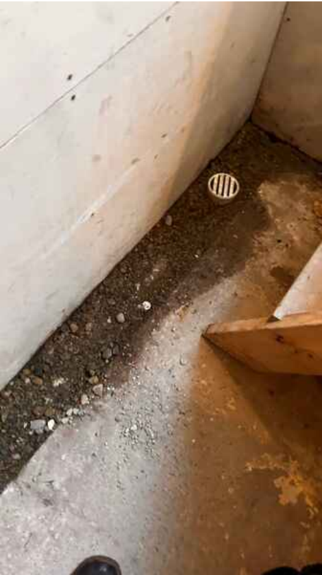
Moisture Noted in Perimeter
