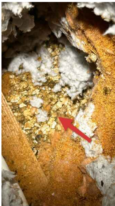
Vermiculite insulation contains asbestos
