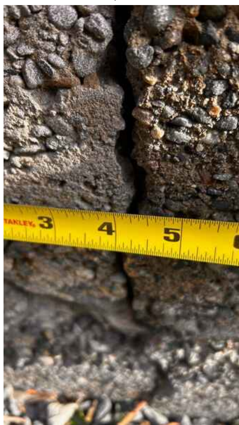
Left side of home crack
