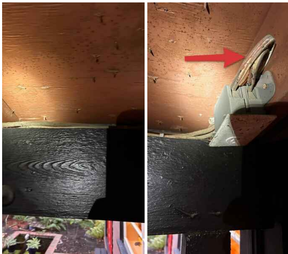
Conductor needs to be BX (protected) or in conduit
