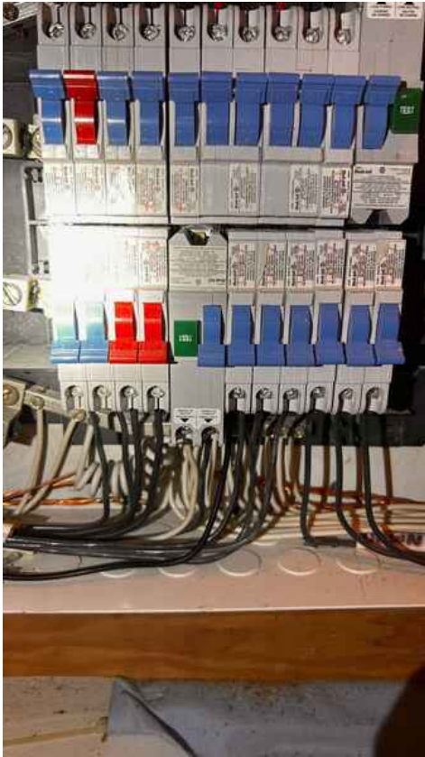
Sub panel photo
