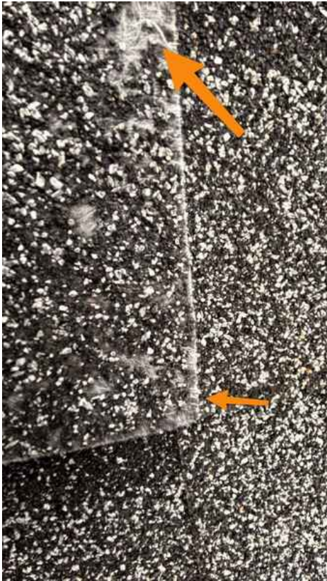
Fiberglass matting visible
