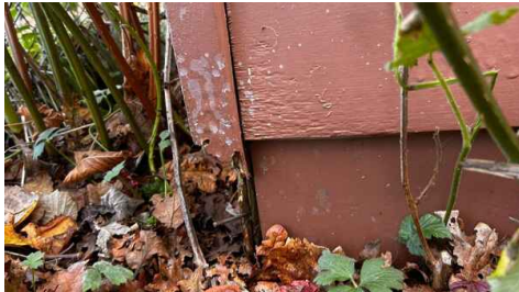
Grade is rotting the siding (garage)
