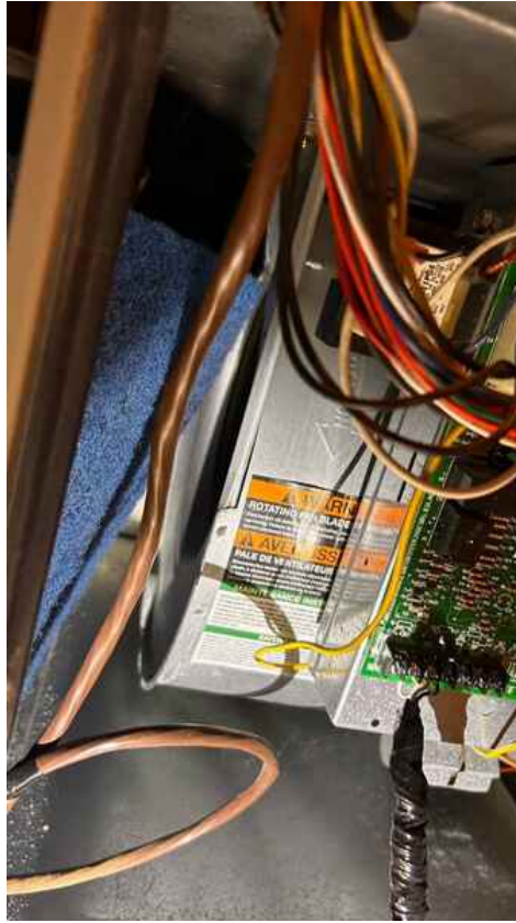
Filter interfering with furnace blower
