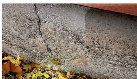
Front crack under porch
