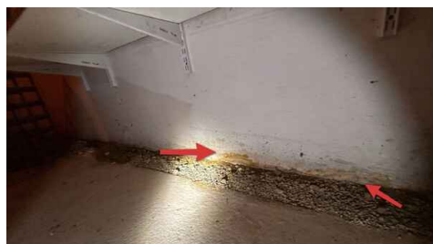
Evidence of moisture in wall material
