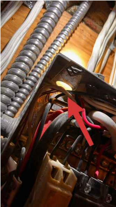
Unprotected opening/ missing knockout
