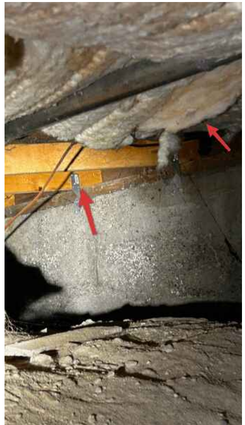
Drooping insulation + evidence of modern joists & clips
