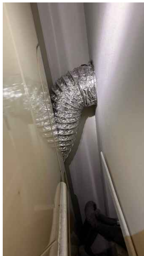
Upgrade to smooth metallic and establish annual cleaning schedule
