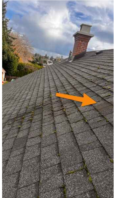
Granular loss (nearly bald shingle)
