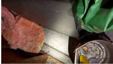
Rodent droppings in garage
