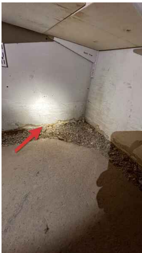
Moisture noted in wall material
