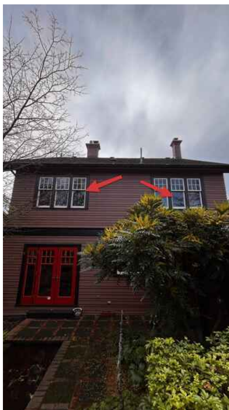
Some windows difficult to operate
