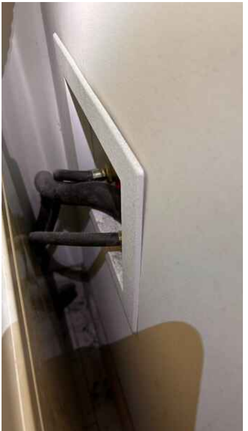
Upgrade to steel braided hoses
