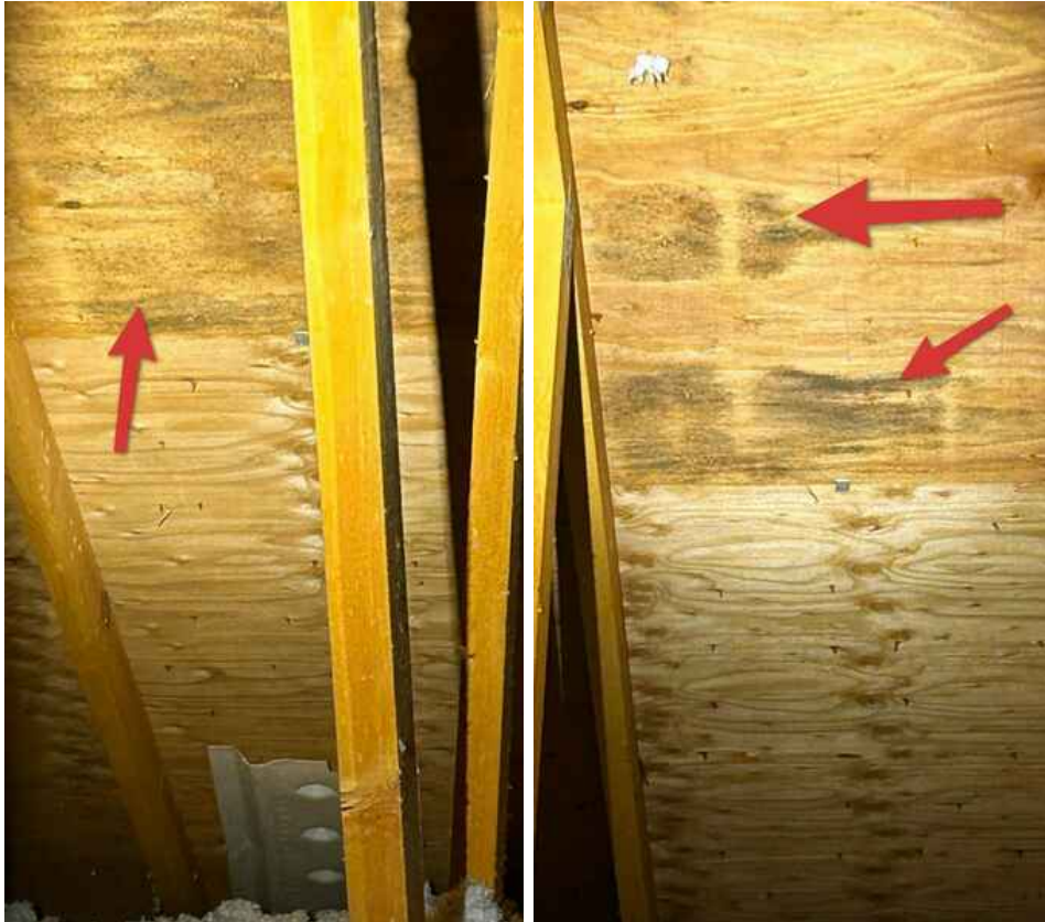
Minor Attic Staining
