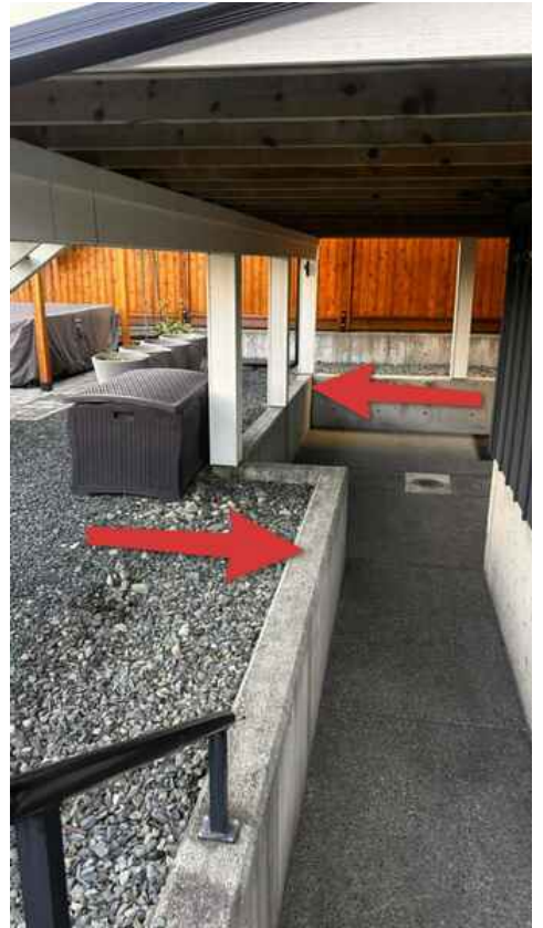
Potential Fall Hazard
