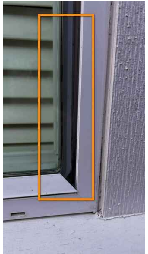
Replace missing window component
