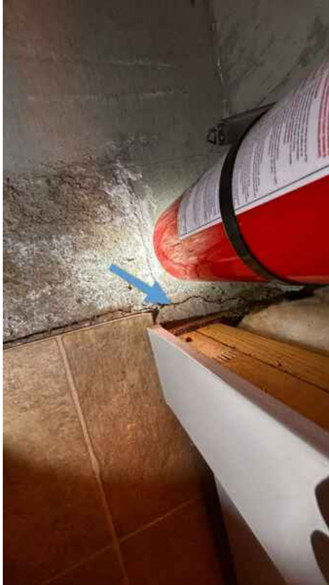
Shrinkage Crack in basement slab
