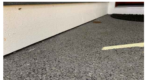
Siding close to ground
