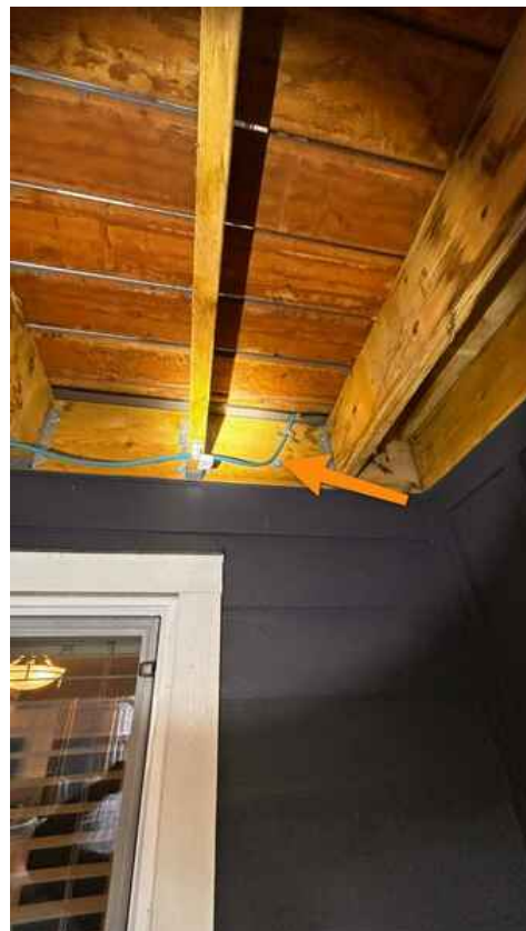
Extension cords not designed to be permanent wiring
