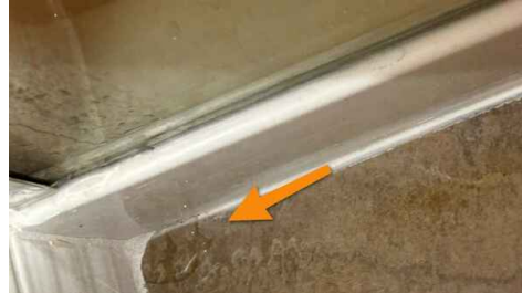
Shower wall not Sealed to tile
