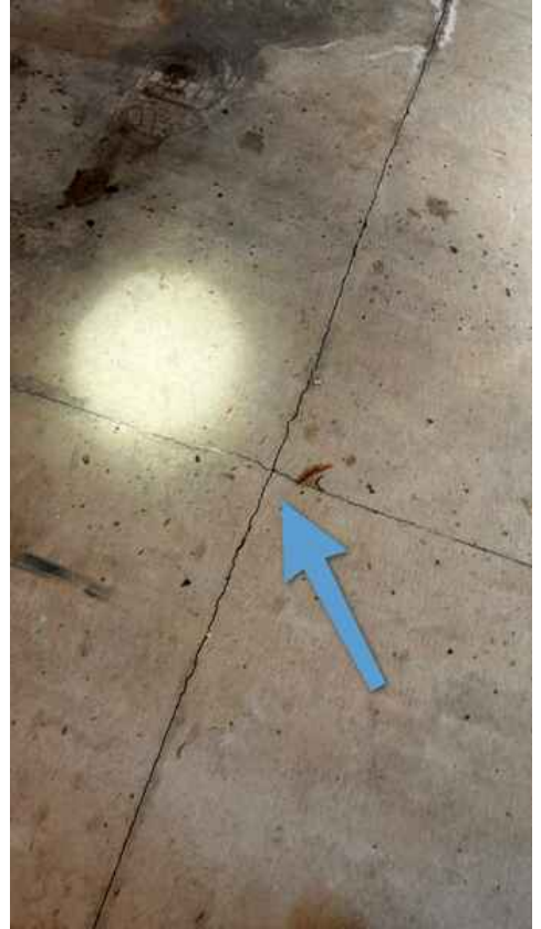
Garage Slab Shrinkage Crack
