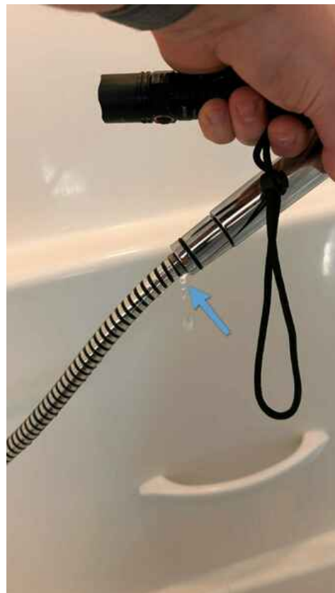
Showerhead leaking slightly
