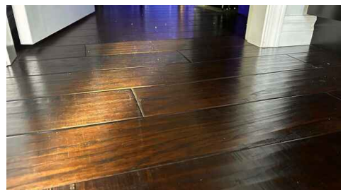
Very Minor Floor Displacement (hard to capture with camera)
