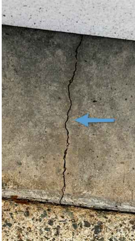
Garage Slab Shrinkage Crack
