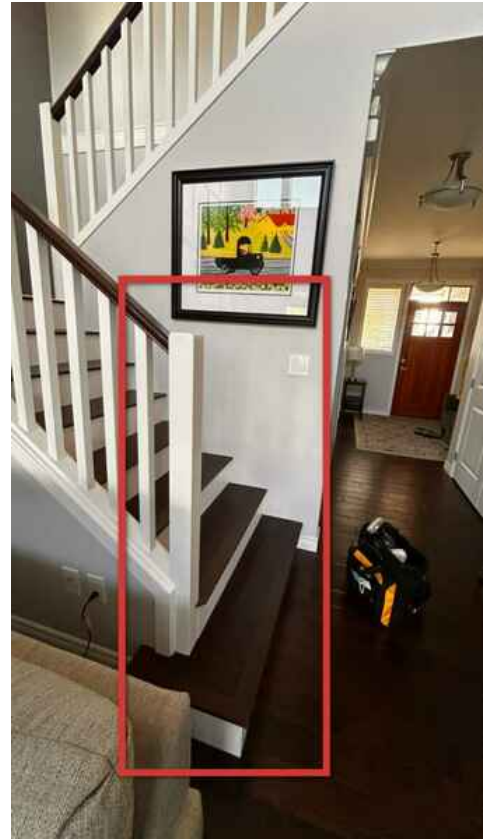
Handrail should extend as far as treads
