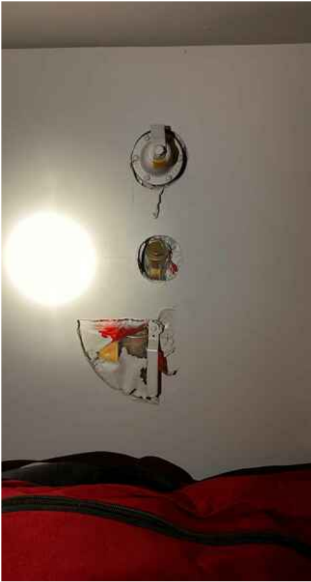
Main Water Shut Off
