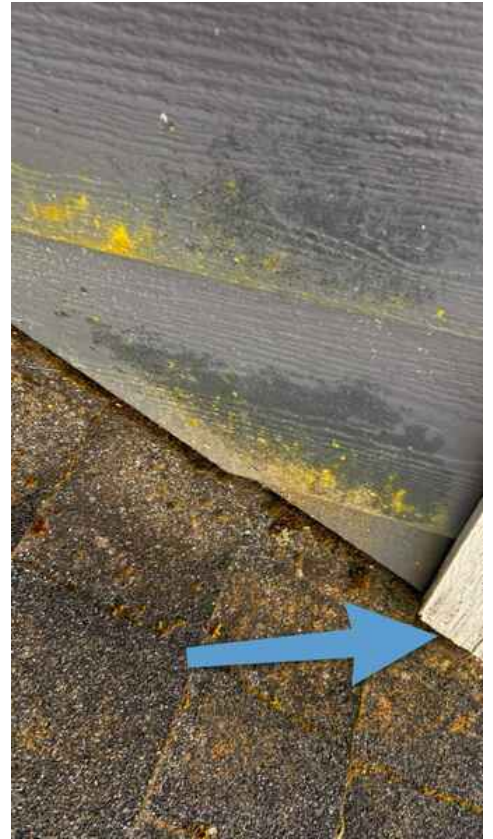
Trim Decay/ Moss
