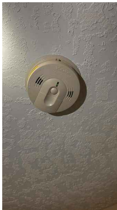
Install adequate smoke and CO detectors
