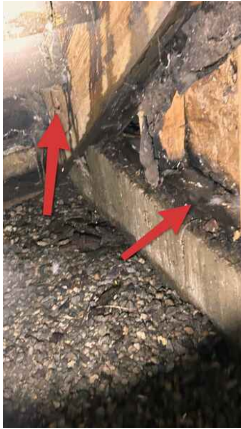
Rotted Stringer, Sill, and Materials
