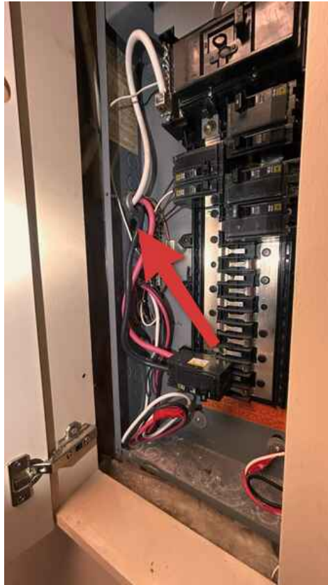
Missing Knock Out
