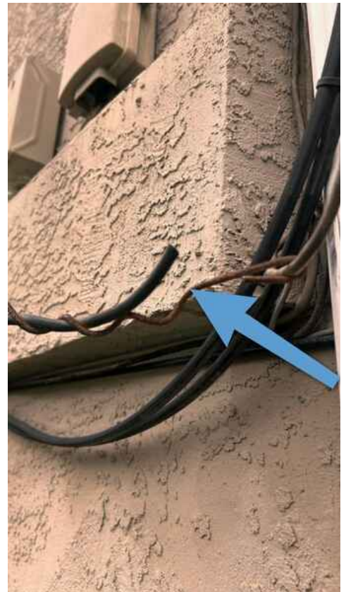
Cable Improperly Terminated
