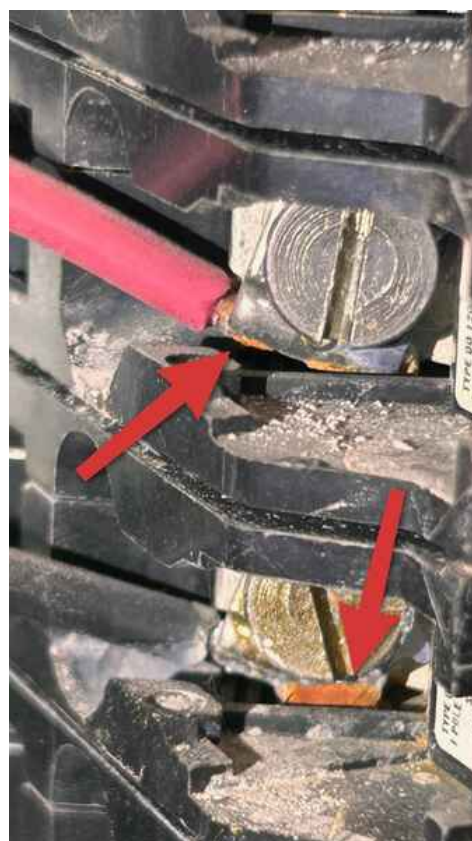
Possible corrosion issue (unit B)
