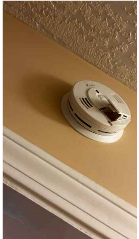
Smoke detector with removed battery (unit A) Very Dangerous!
