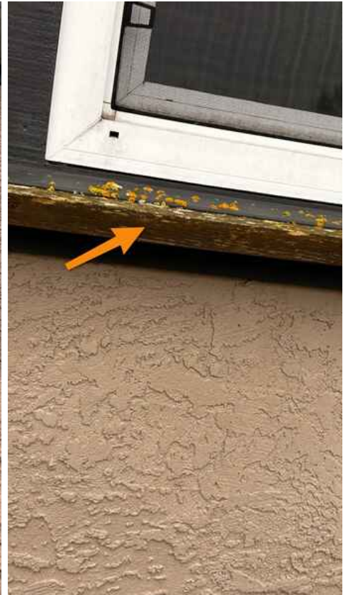
Rotted Sills throughout
