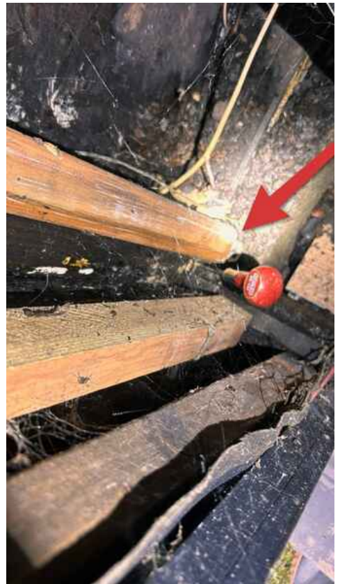
Rotting Sill/ Structure
