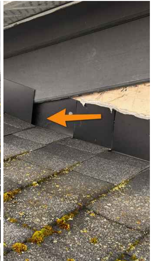
Gap in step flashing
