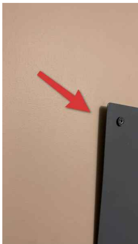
Cover screws don't hold tight (unit C)
