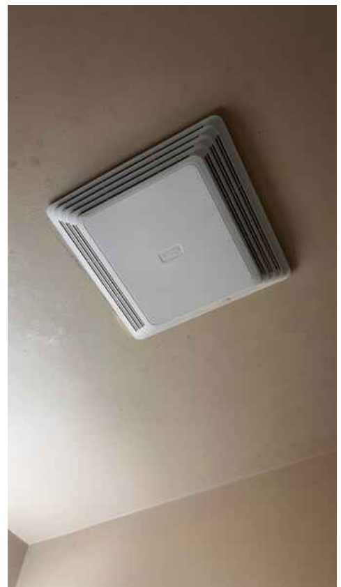
Inefficient Bathroom Fans
