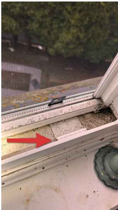
Water pooling in track
