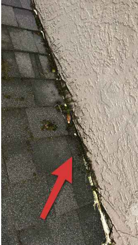
Missing step flashing, visible discoloration
