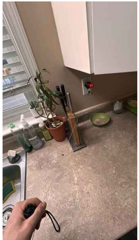
Kitchen not GFCI protected
