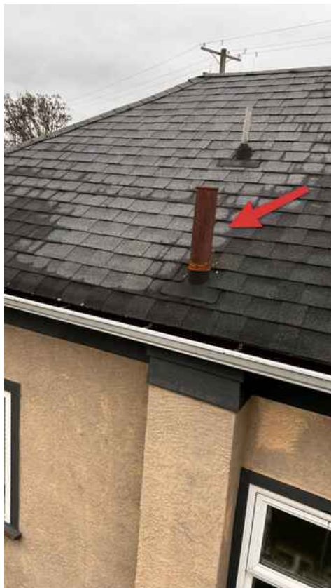
Cast iron Vent
