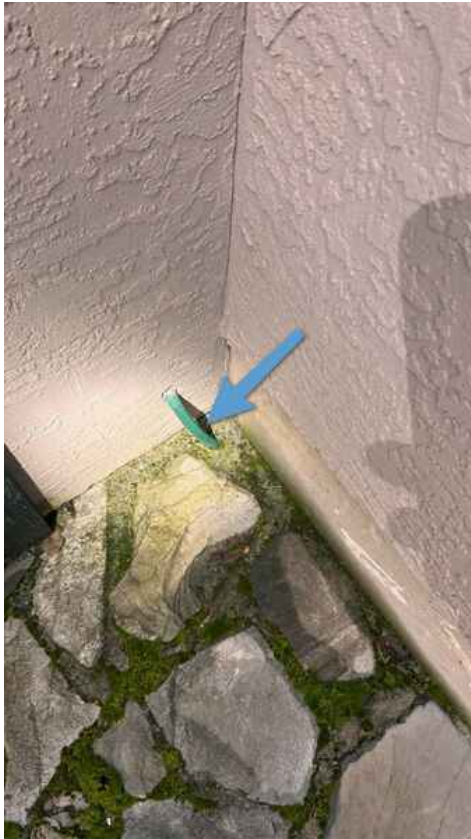
Garden hose under grade
