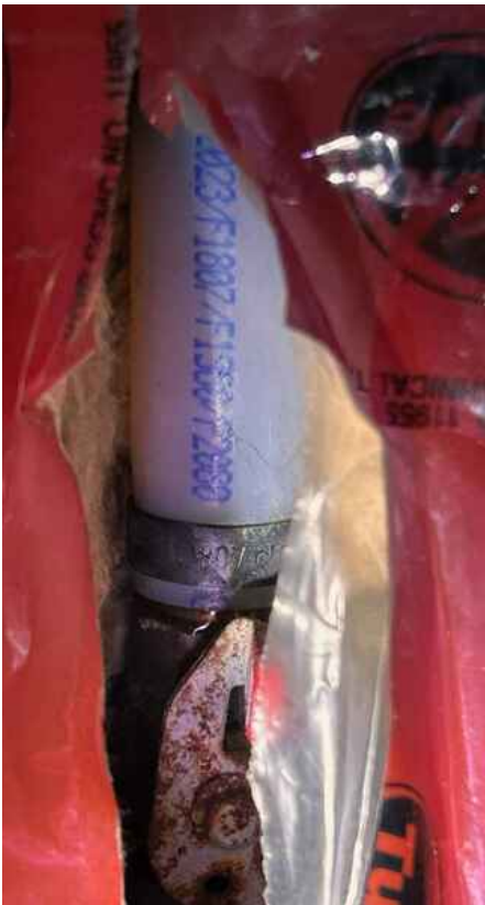
Main water shut off
