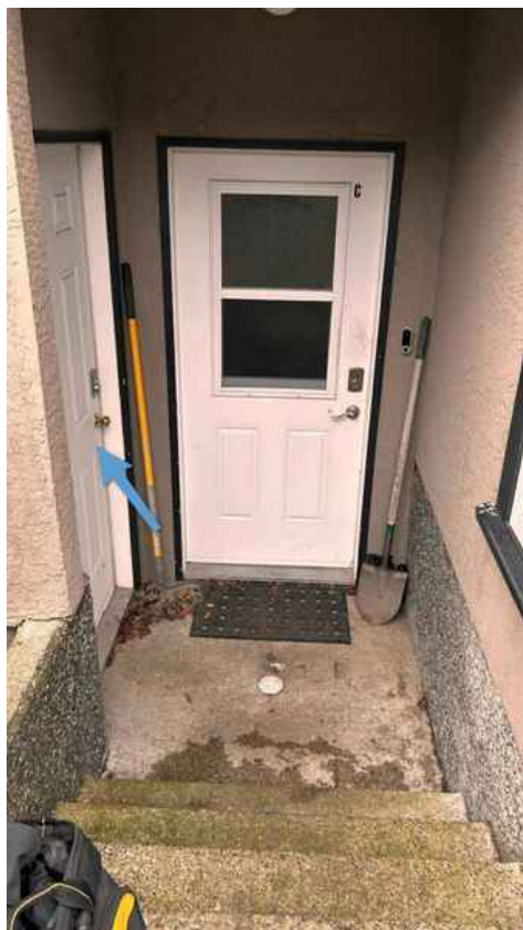
Utility room door doesn't latch
