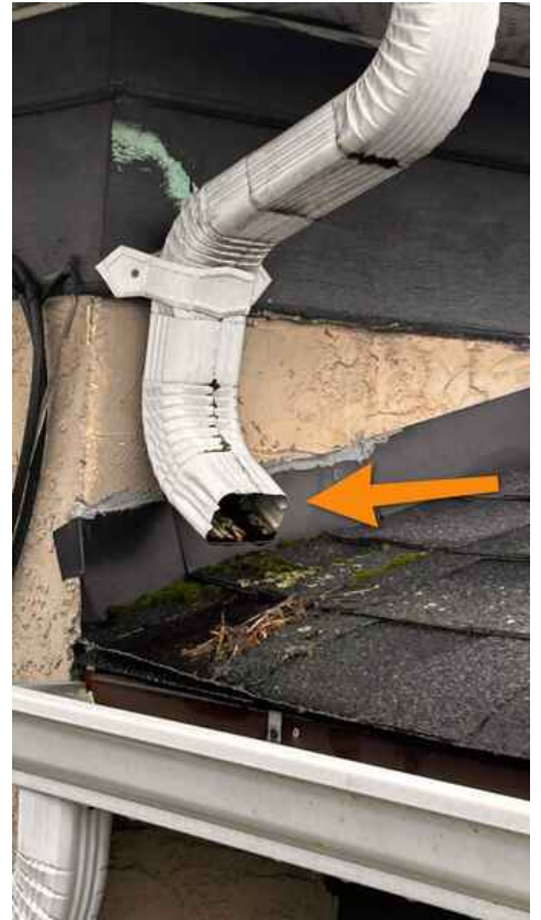
Extend downspout to gutter
