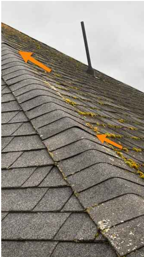
Slightly lifted shingles
