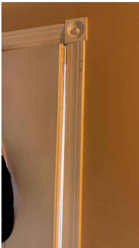
Misaligned Door (unit A)
