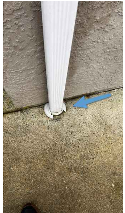
Chipped/ Broken covers
