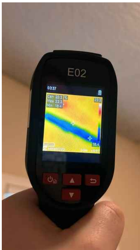
Thermal image of ceiling (cold spot tested dry)
