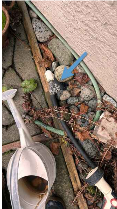
"temporary" hose bib Not winterized
