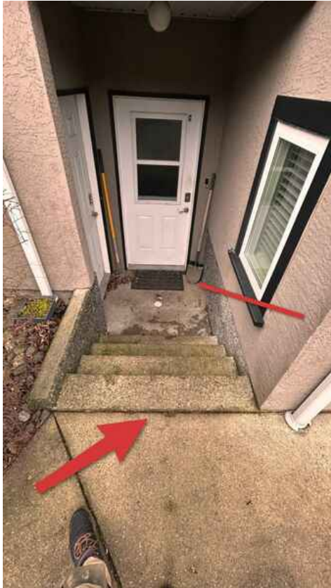
Missing handrail & Trip Hazard
