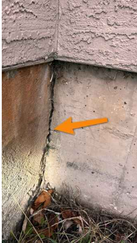
Crack, Differing concretes
