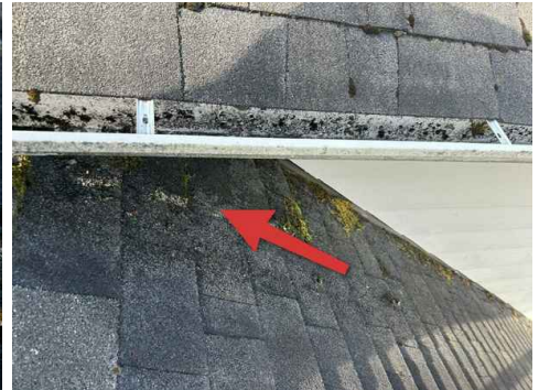
Gutter draining directly onto roof surface
