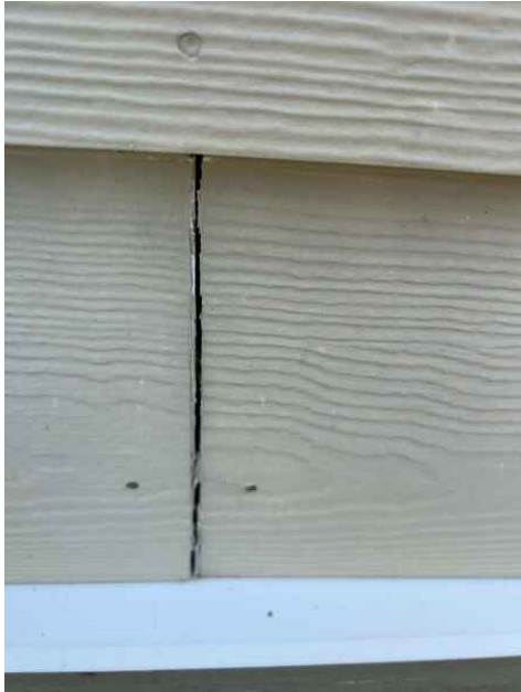
Caulk Gap in siding
