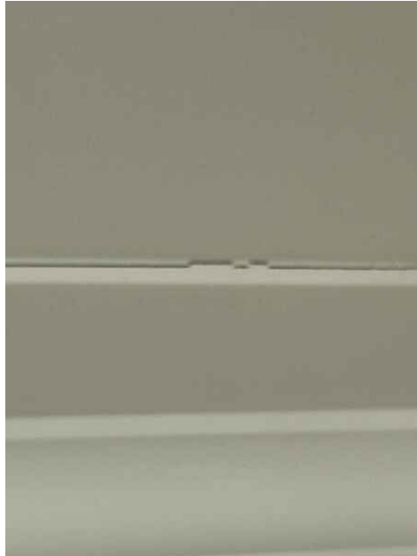
Crown Moulding Separated
