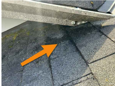
Premature Shingle Wear, Add Downspout
