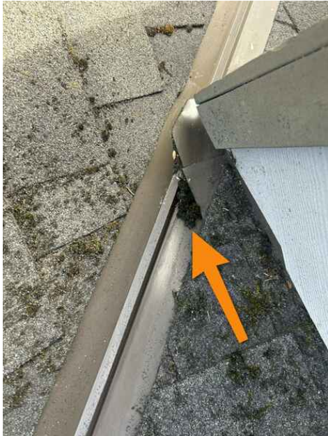
Valley Flashing Running Through Step Flashing
