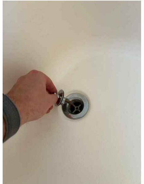
Tub stop not attached
