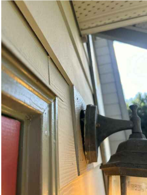
Light fixture exposed
