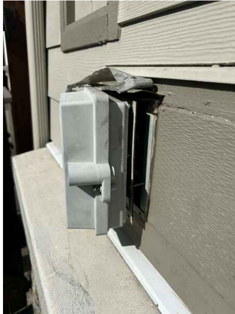
Damaged Telecom box
