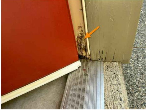
Door Frame Damage
