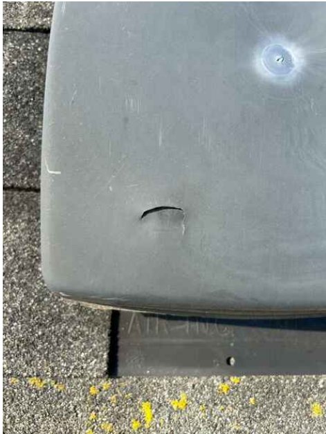
Cracked Roof Vent
