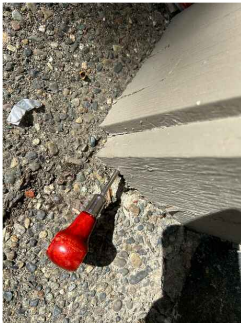
Garage Trim Slightly Rotting
