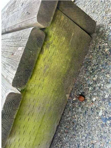
Signs of rot/decay
