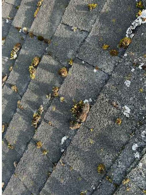
Moss build up
