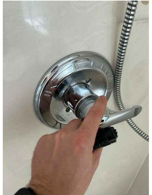
Faucet Control Was loose
