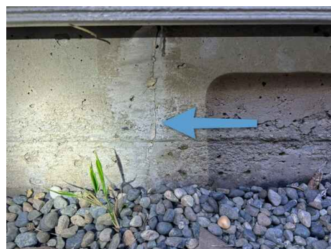
Minor Shrinkage Crack
