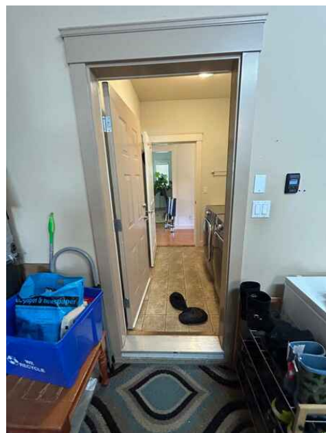
Man door needs to self close
