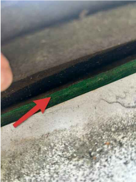
Missing Drip Edge Flashing
