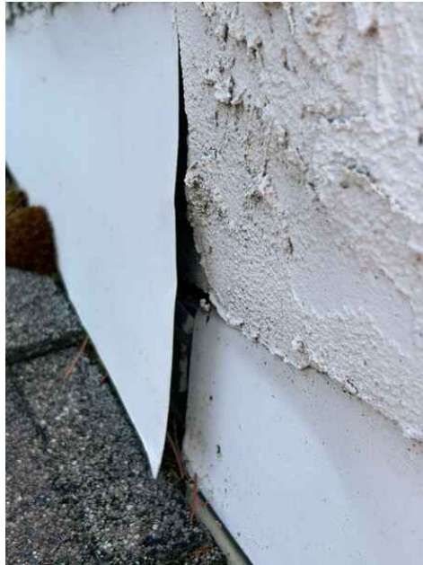
Counter Flashing bent
