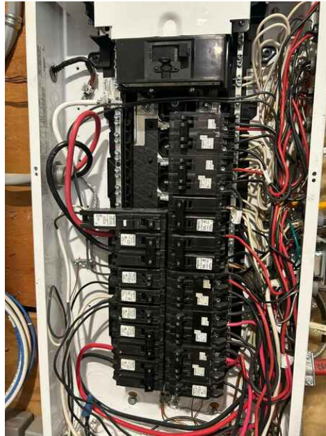
Panel with cover removed
