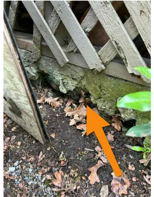
Undermined Patio Slab Due to Grading
