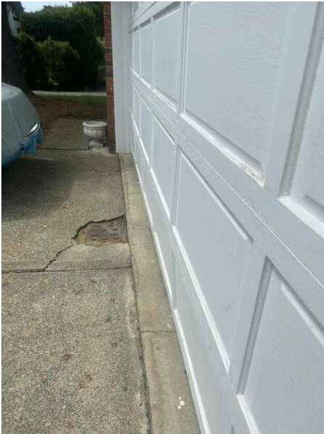
Bowed Garage Door
