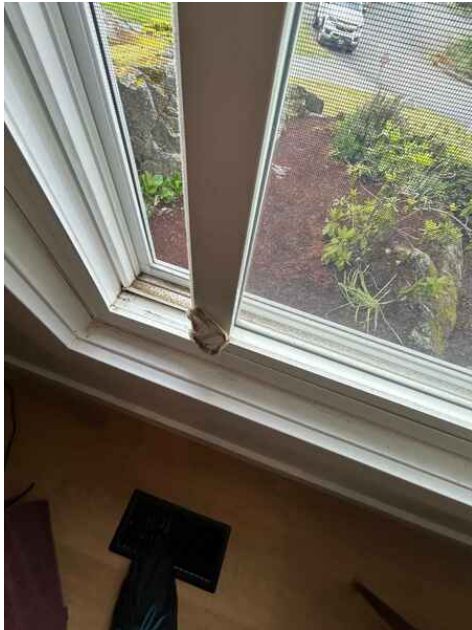
Weather stripping broken/ Sticky window
