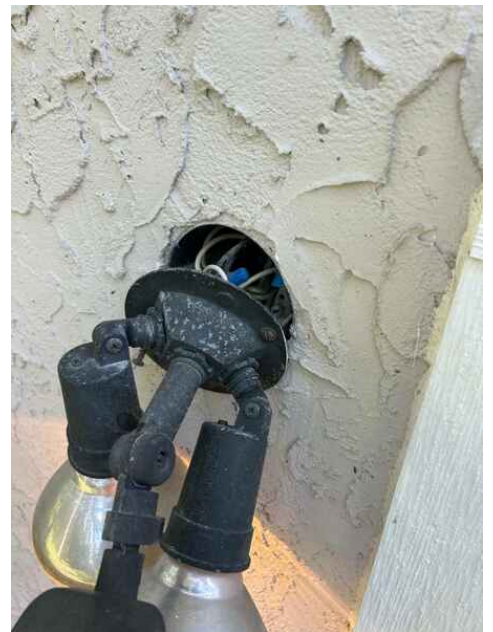
Fix light fixture
