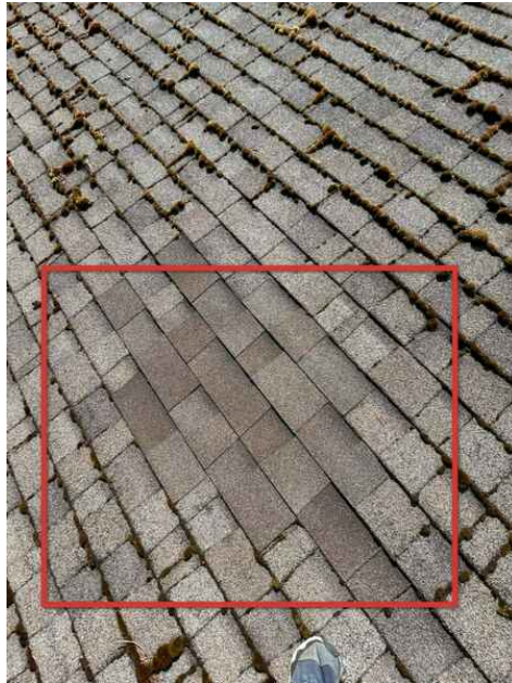
Evidence of a previous patch
