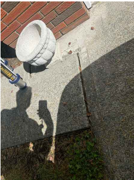
Brick siding too close to grade
