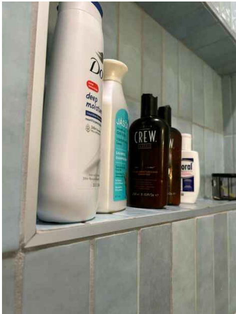
Flat Sections hold Water
