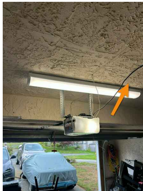
Garage motor plugged into extension cord
