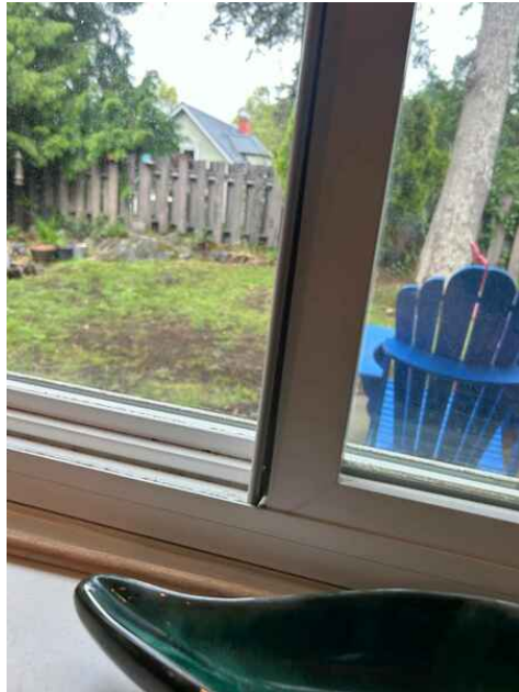
Broken/ worn component
