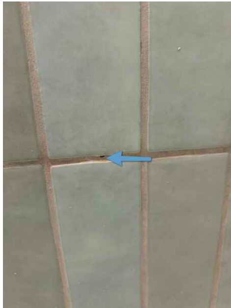
Pin hole in grout
