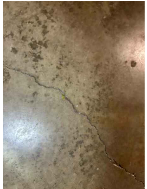
Cracks in Garage Slab
