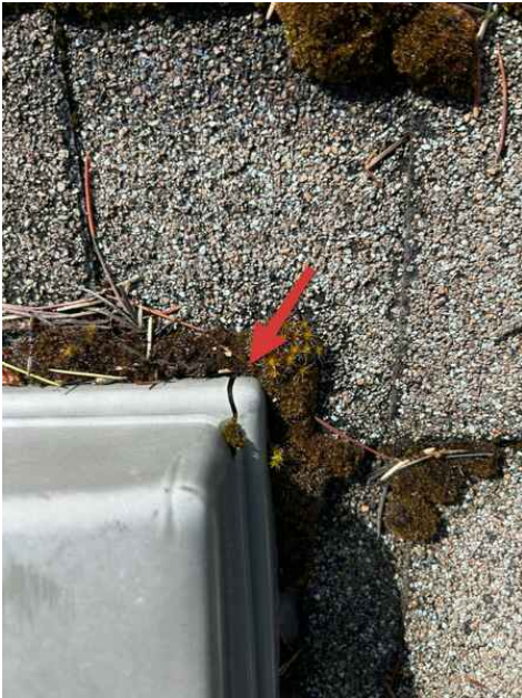
Cracked Vent Casing
