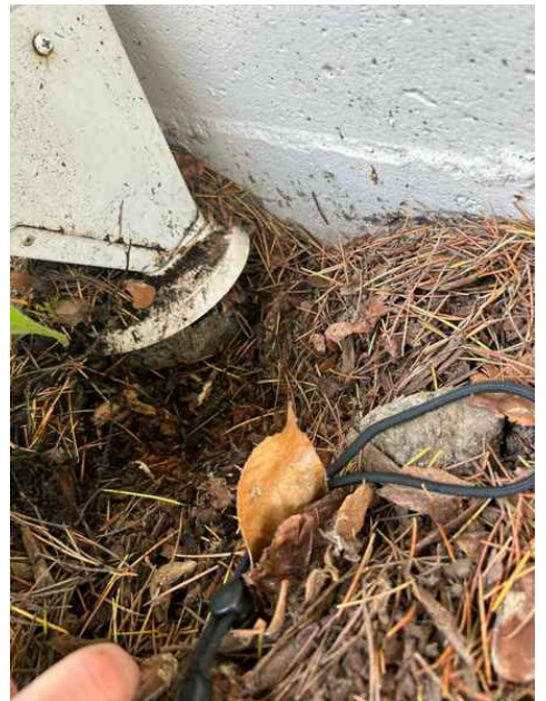
Concrete tile drain
