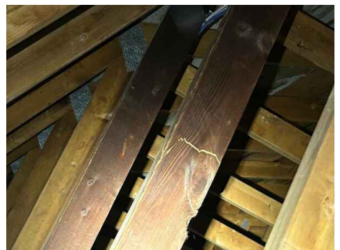
Cracked Truss Member
