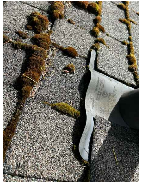
Warped Vent stack boot
