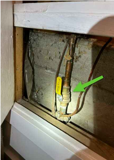
Main water shut off
