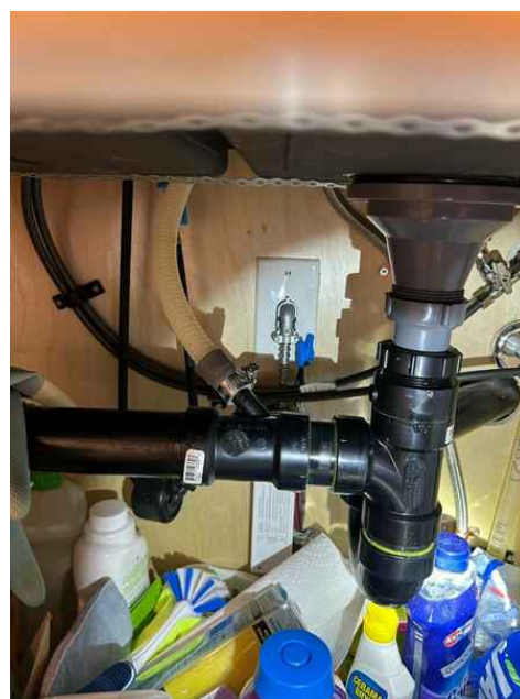
Put open connection in junction box (high humidity area)
