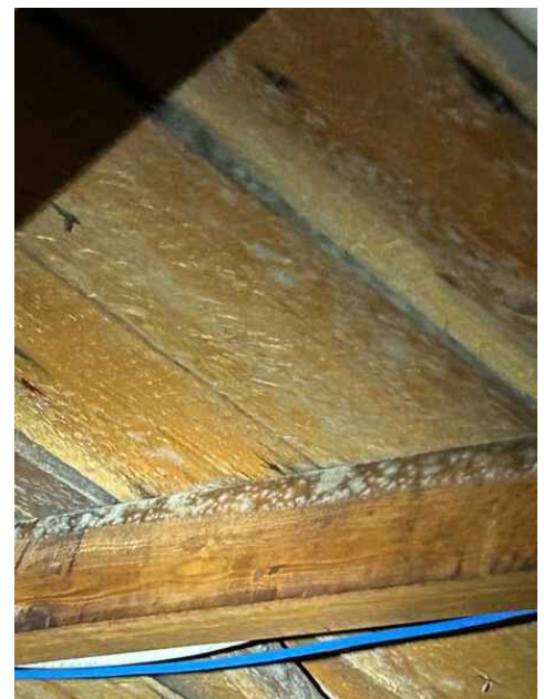
Staining on attic structural members
