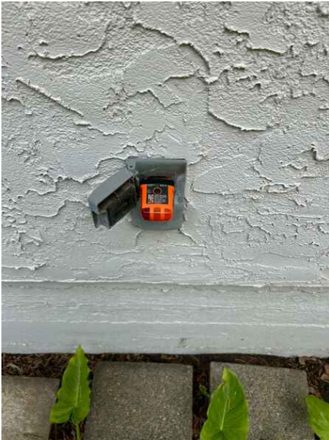
Majority of exterior outlets not GFCI protected
