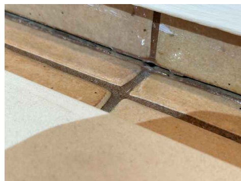
Behind kitchen sink needs caulk/silicone
