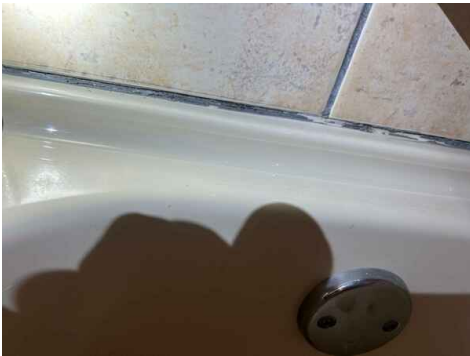
Missing caulk/ silicone
