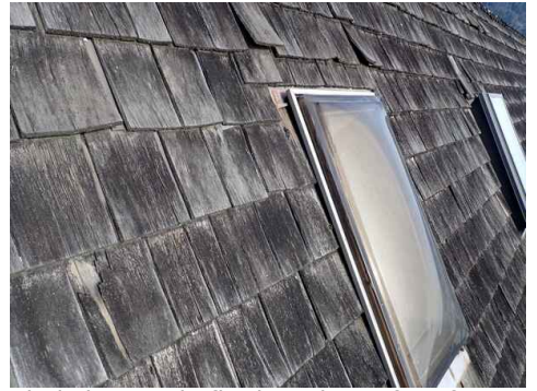
Skylight nearly flush with roof surface
