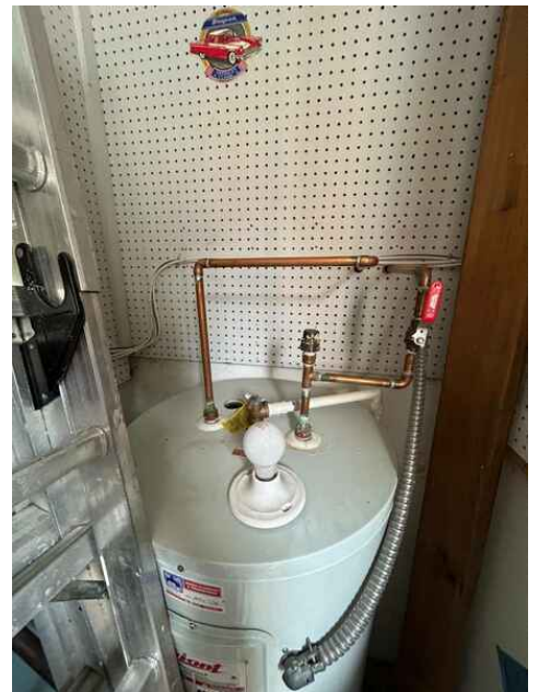
Missing expansion tank
