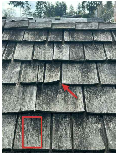
Lifted and split shakes
