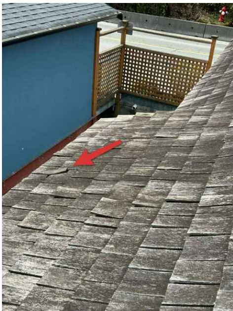
Broken loose and missing sections
