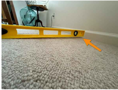
Floor not level in short span
