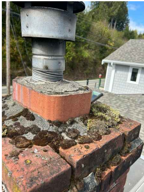
Missing cap increasing water ingress
