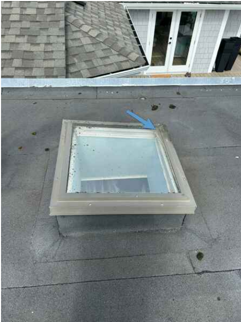
evidence of pooling on skylight
