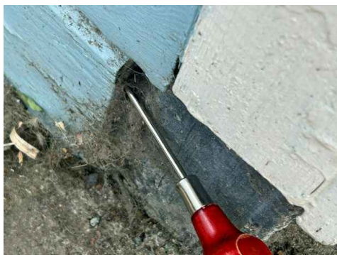
Siding boards showing signs of rot
