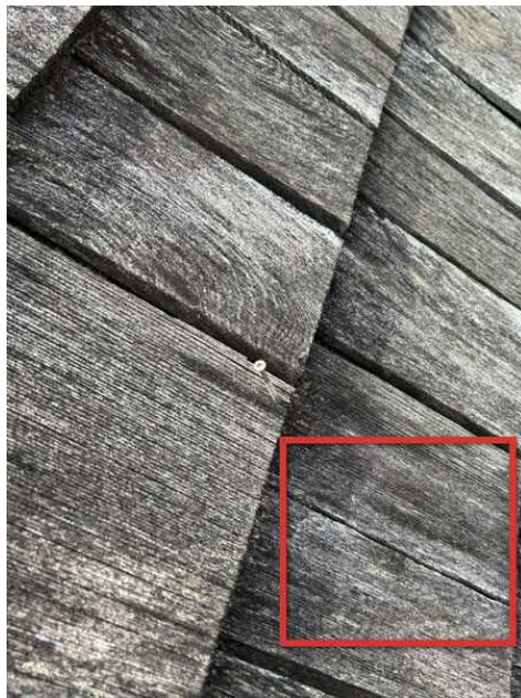
Multiple split shakes throughout
