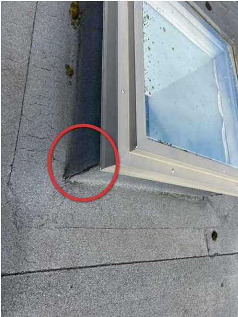
Split material on skylight curb
