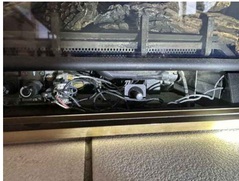
No shut off valve at unit
