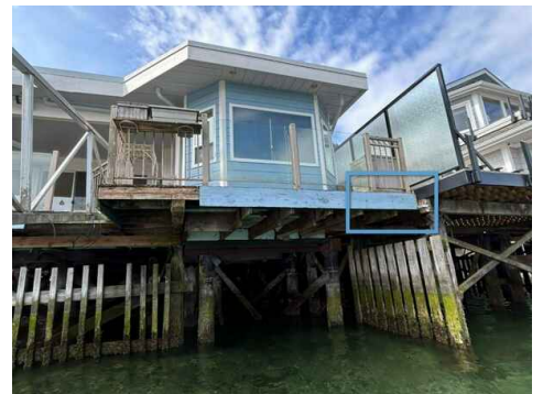
Section of fascia falling off
