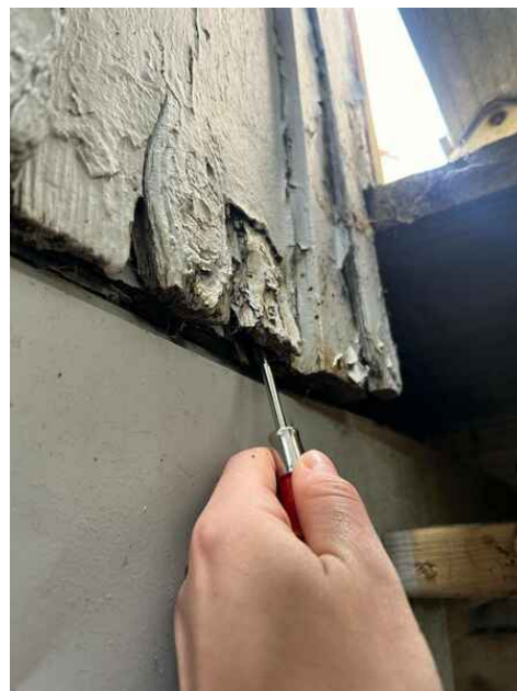
Severe Rot on Right lower siding
