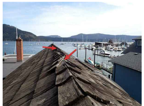
Ridge line damaged
