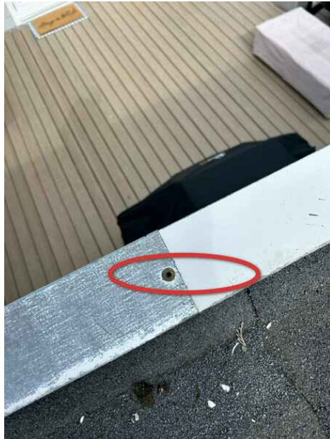
Rusted exposed hardware
