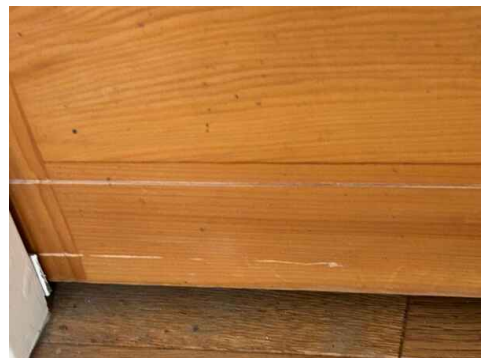
Pocket door to coat closet is scraping
