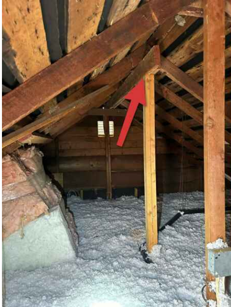
Rafters taken out and attempted replaced load
