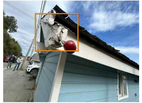
Very rotted fascia
