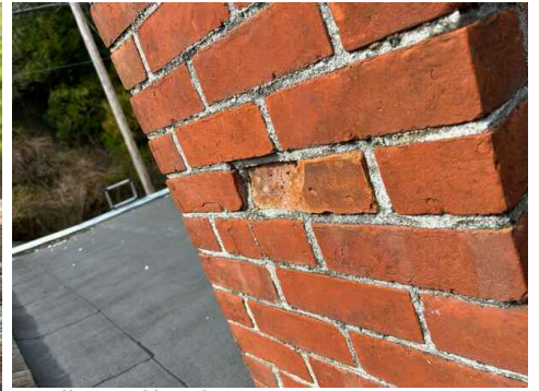
Spalling of bricks
