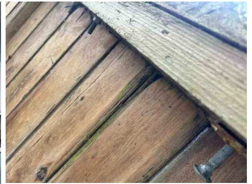
Hardware insufficiencies for walkway
