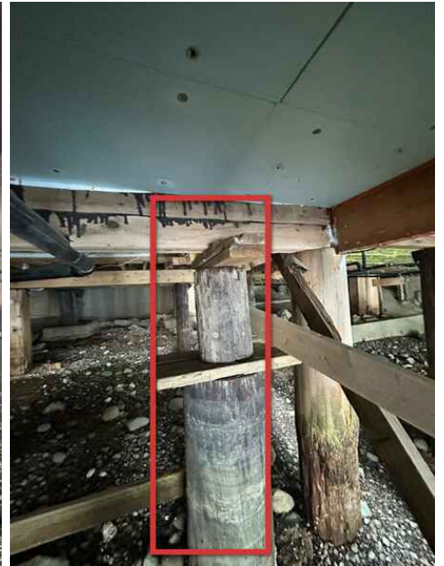
Improper building practices, Log to shim to log to shim
