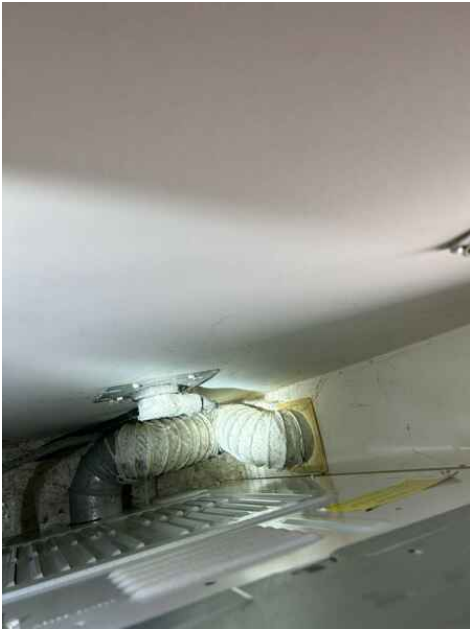
Non metallic corrugated tubing is unsafe
