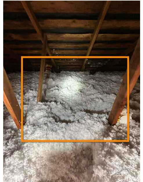
Compacted insulation in attic due to work
