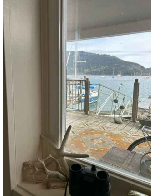
Failed seal rear windows
