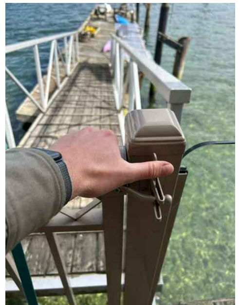
Gate and latch out of alignment
