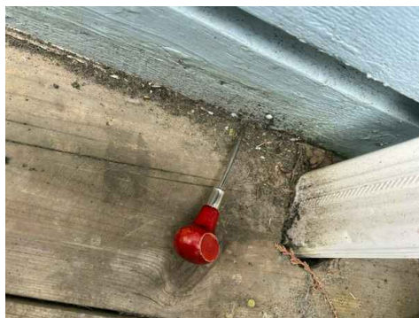
Soft wood noted near car park area
