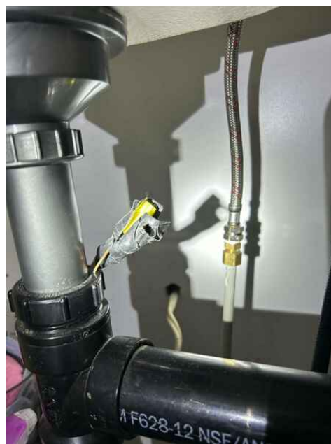
Wiring should be completely removed
