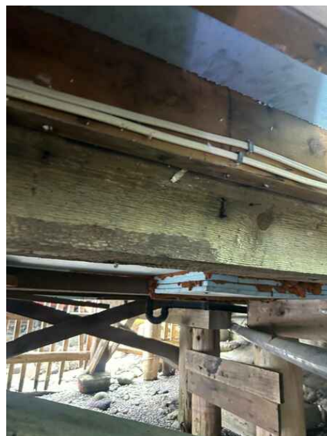
Interior wiring used outside
