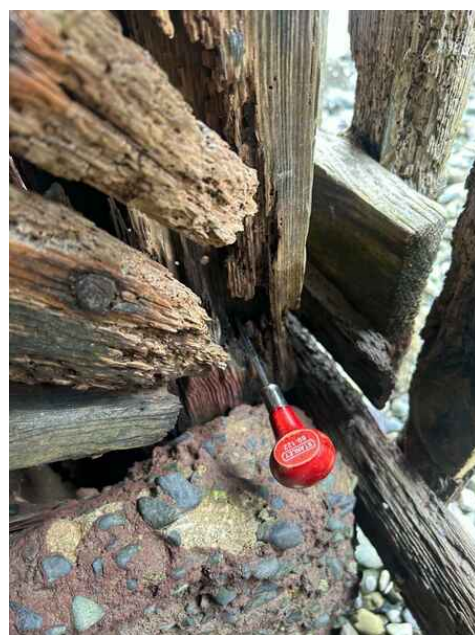
Severely rotten posts in degraded footings
