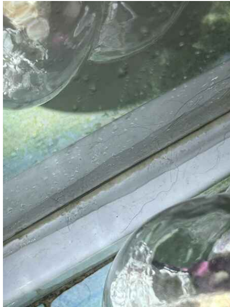
Needs caulking maintenance
