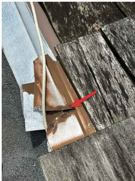
Voids and deteriorated flashings throughout
