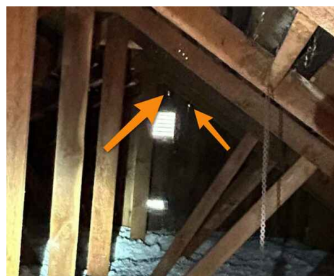
Penetration of light near gable vents
