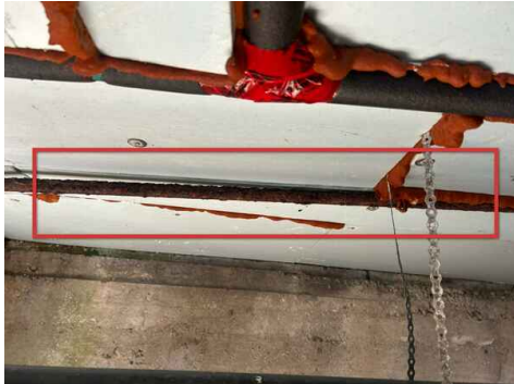
Gas line corroded
