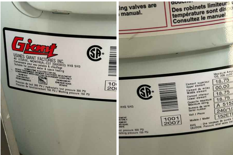
Water heater well past life expectancy
