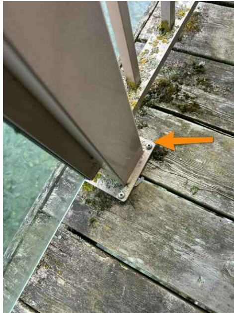
Apply mastic to hardware to prolong, and fix deck boards to secure gate
