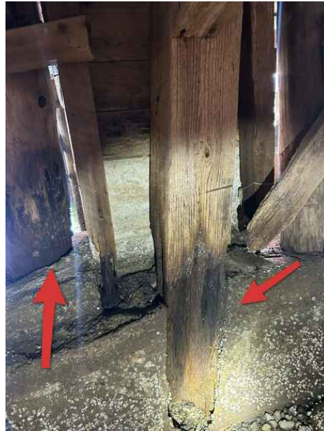
Severe rotted support post in disappearing footing
