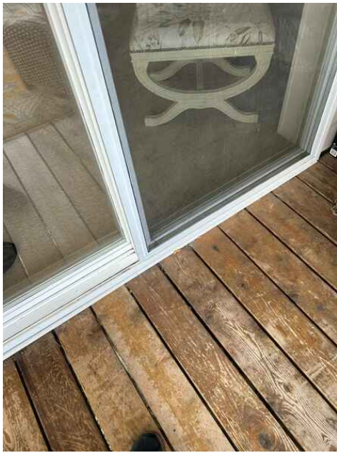
No flashing observed
