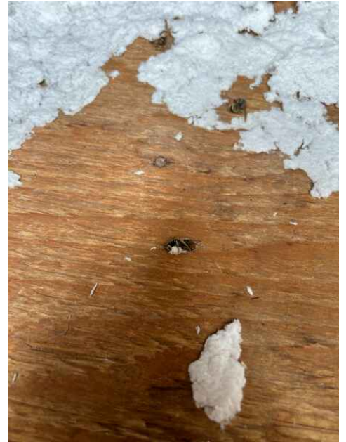
No visible vapor barrier
