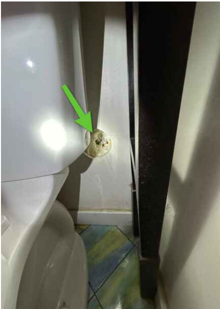
Possible main water shut off
