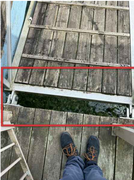
Large gap to walkway (fall hazard)
