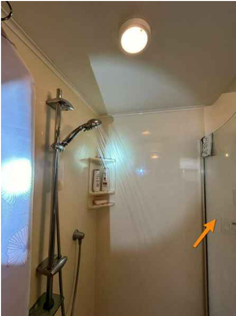
Glass partition leaking
