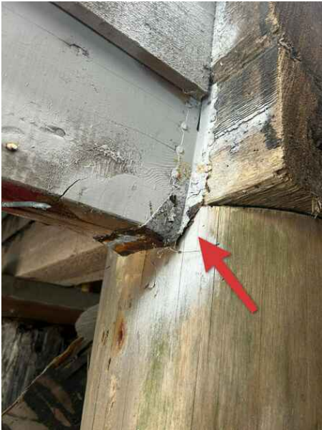
Beam used with joist hanger, insufficient end bearing
