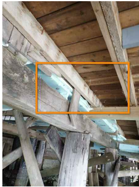
Missing flashing underneath deck, will lead to water ingress of the insulation assembly
