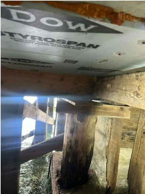
Shims used over post log in a deteriorated footing
