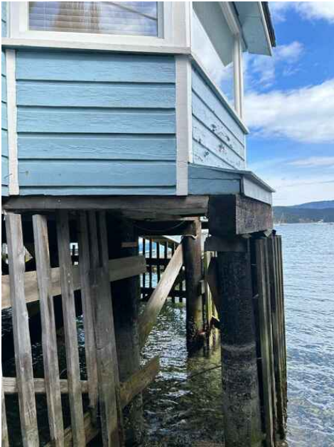
Section of home is obviously displaced inside
