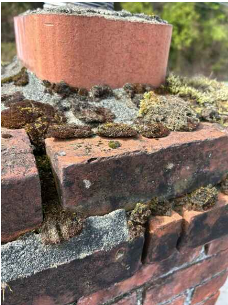
Missing cap and serious voids
