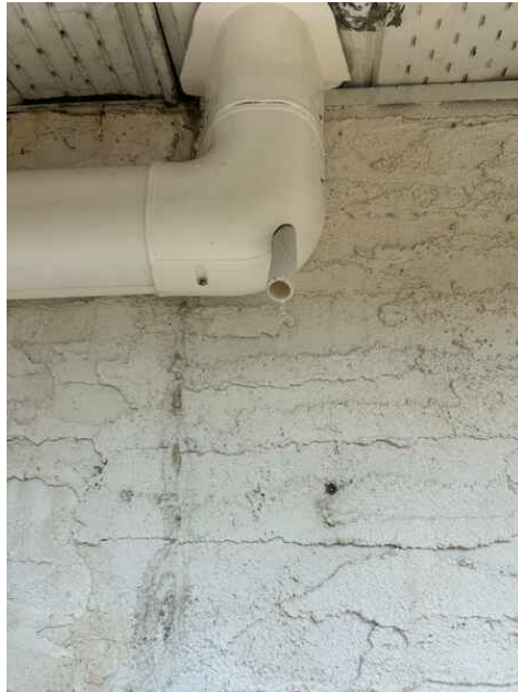
Condensate drain close to home (annoyance)
