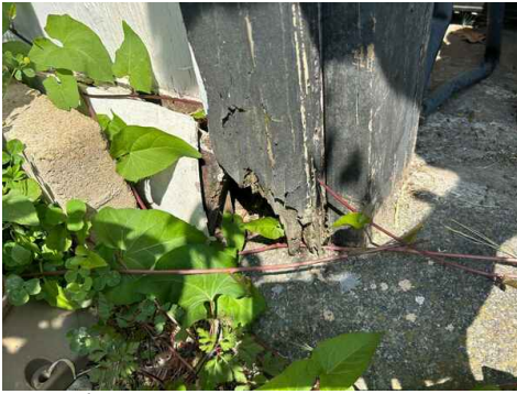
Rotted trim (garage)
