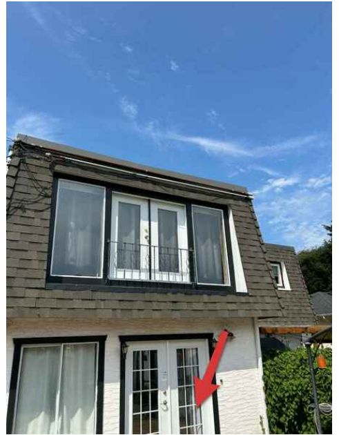
Unable to open 1 french door lock
