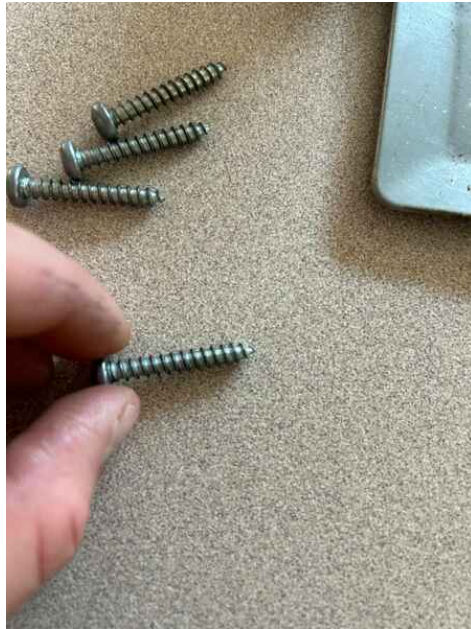
Improper screws securing panel (sharp tipped)
