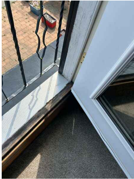
Difficulty opening juliet doors
