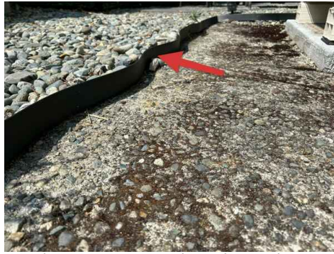
Landscaping material trip hazard
