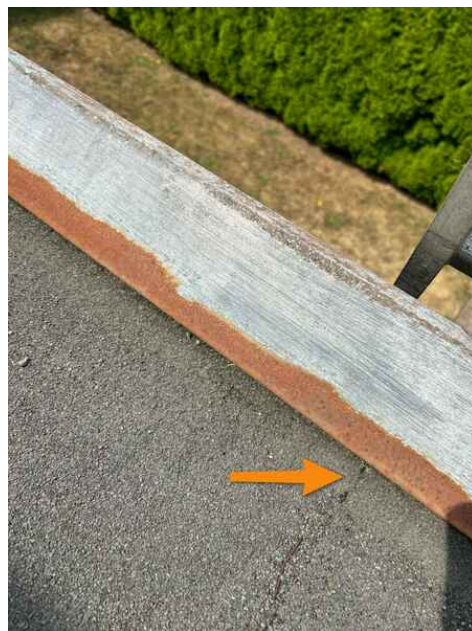
signs of granular loss and pooling
