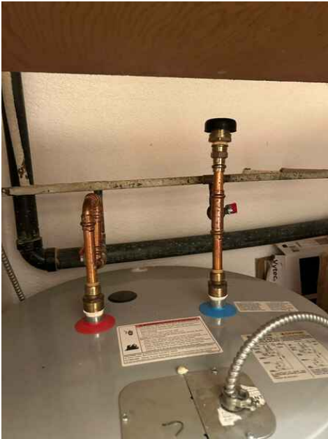
Missing expansion tank
