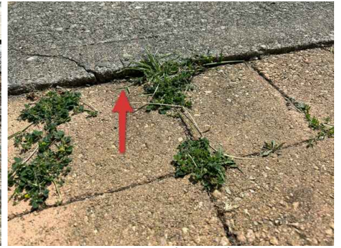
Concrete/Paver trip hazard
