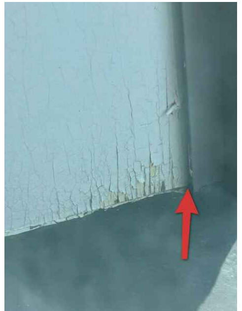
Possible entry point for water due to deep window well design
