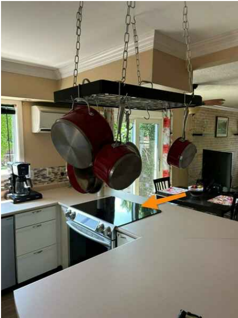
Lack of kitchen exhaust
