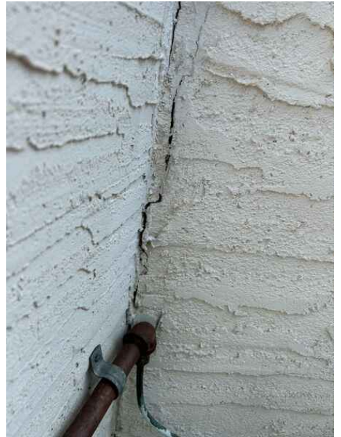
Cracking near chimney
