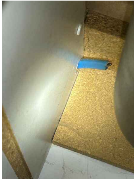
Stray conductor under sink (not tested)
