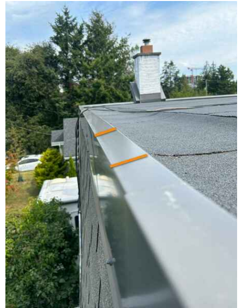
Some sections of parapet flashing are sloped incorrectly
