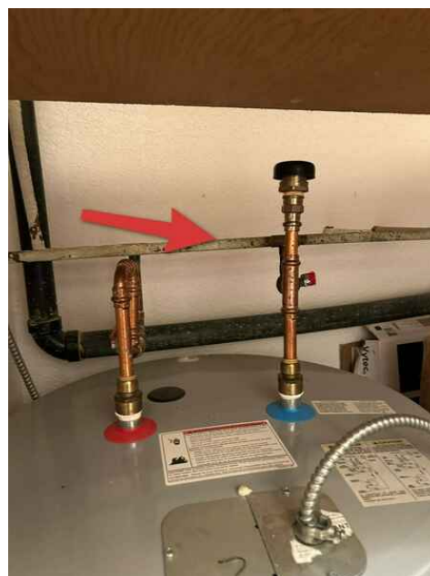
Ageing copper pipes throughout home
