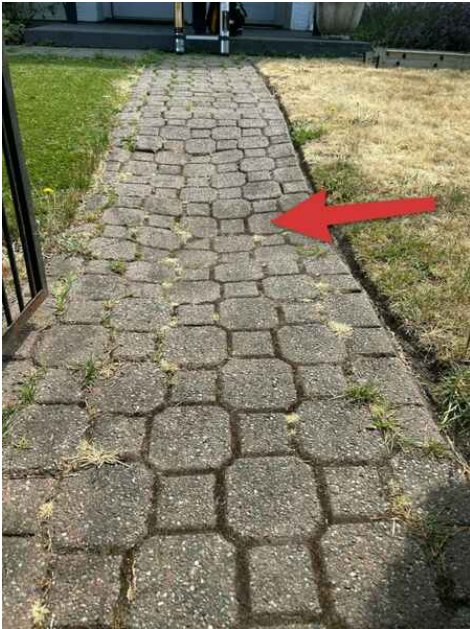
Paver trip hazard
