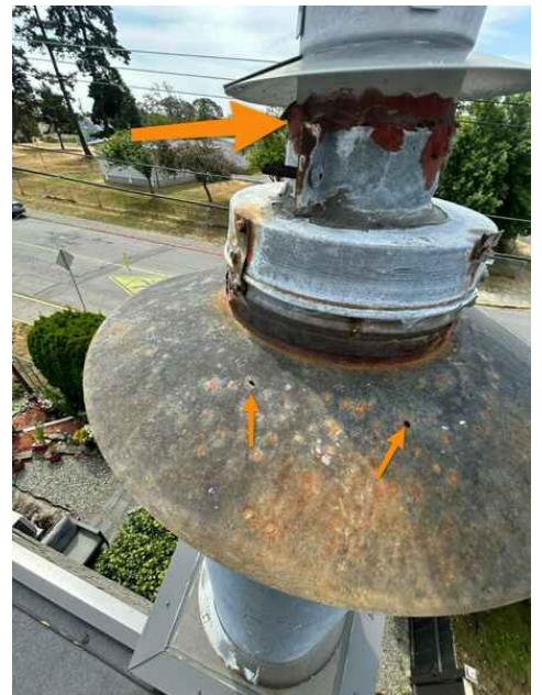
Rusting and pitted rain guard
