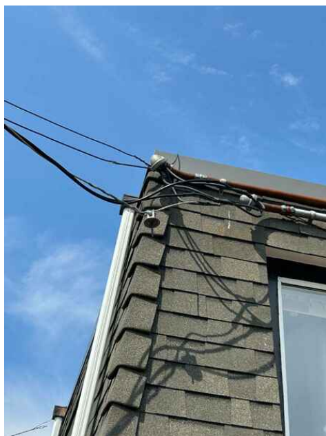
Other occupants of duplex are also responsible
