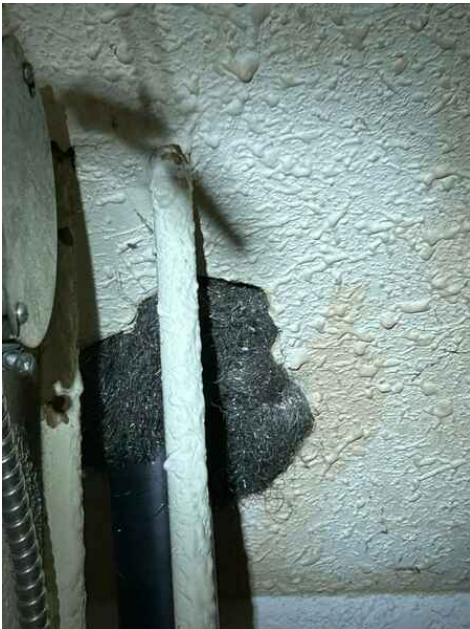
Steel wool used in living space as deterrence.
