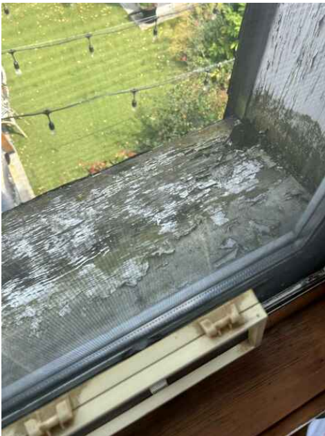
Severely Rotted Sill
