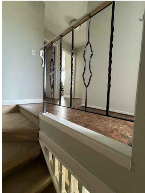
un-sturdy guard rail, wide balusters
