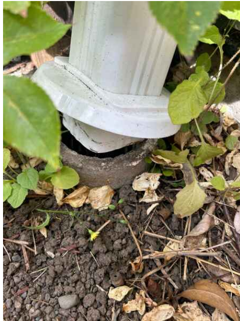
Scope for blockages/collapse
