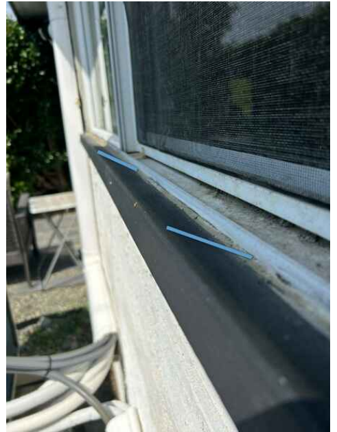
Negative sloped sill
