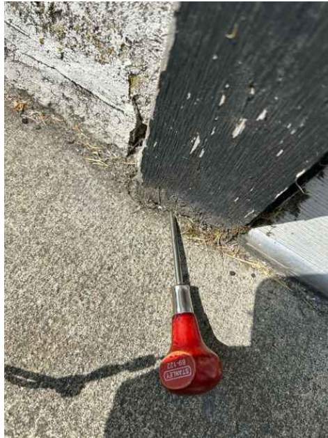
Trim decaying due to contact with grade
