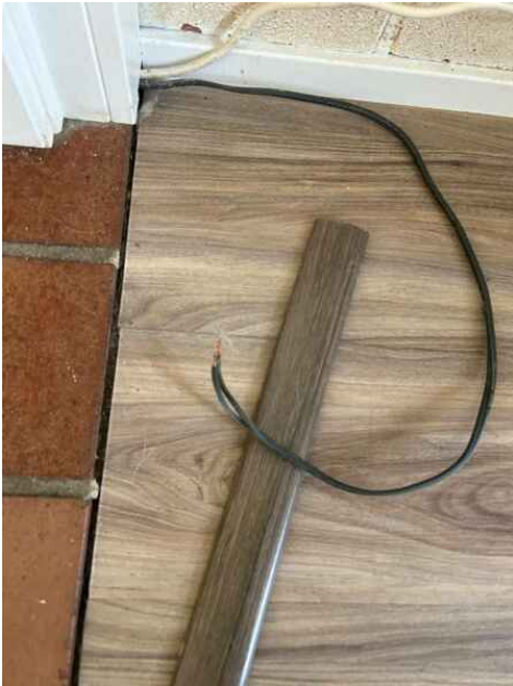
Stray conductor near fireplace (tested dead)
