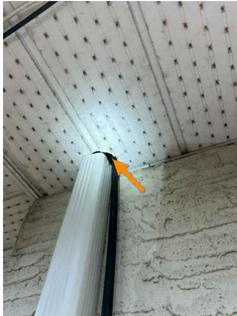
Gap where downspout meets soffit
