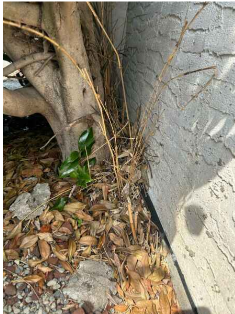
Tree very close to slab
