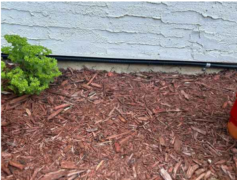
Siding too close to grade
