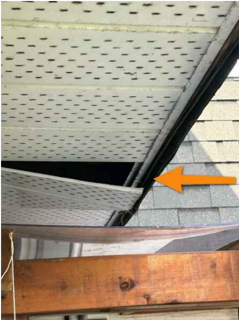
Major Gap in Soffit
